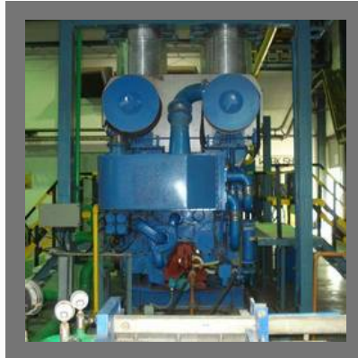
Industrial Diesel Generator Set
